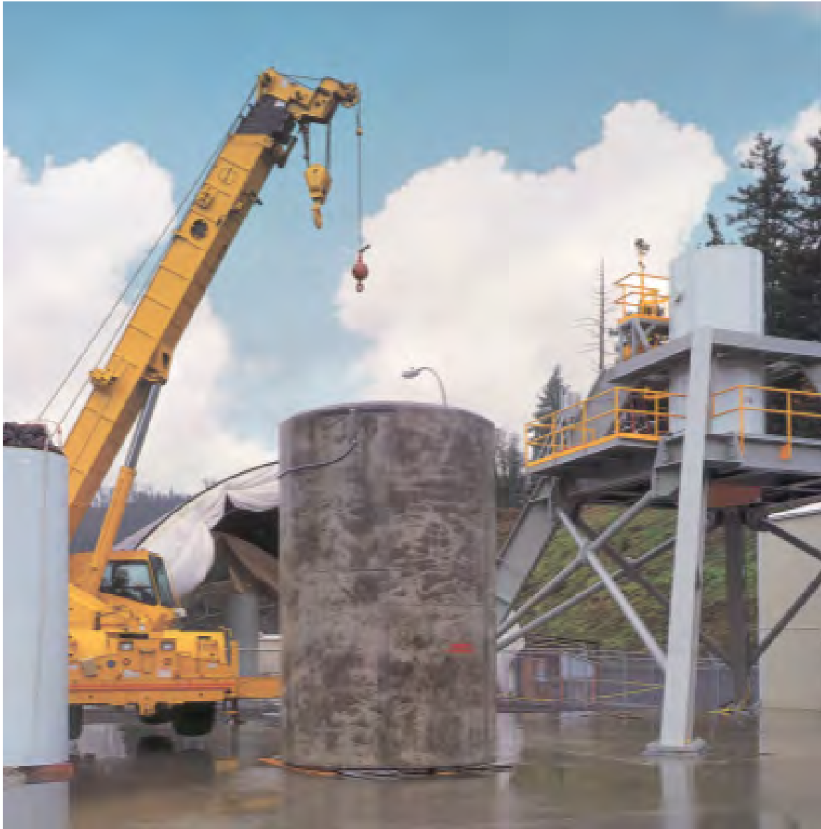
Figure 3.2-6 Holtec MPC-24E Canister in a TranStor Storage Overpack at the Trojan ISFSI
