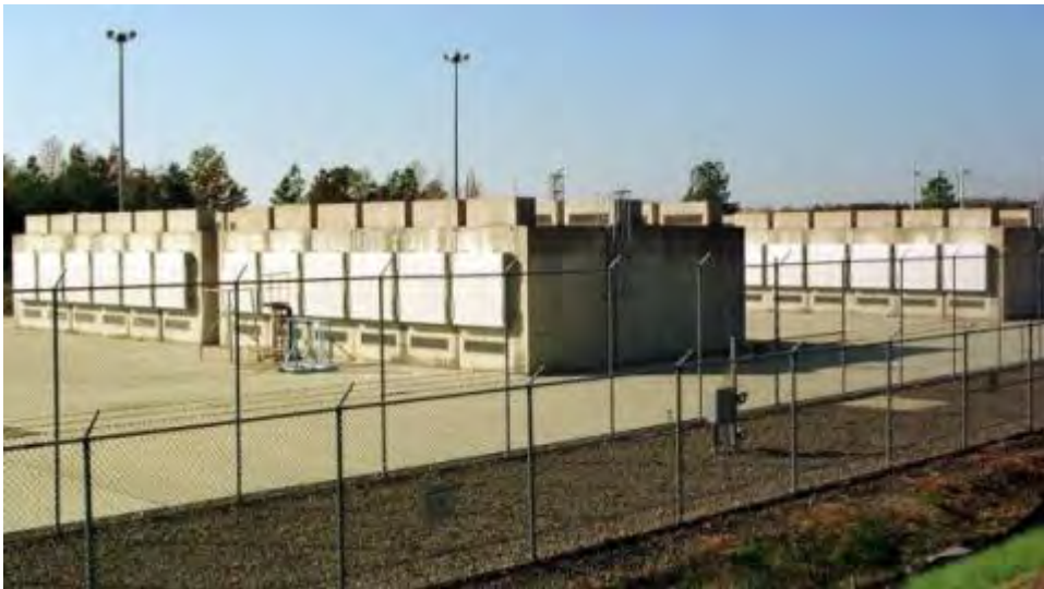
Figure 3.2-45 NUHOMS 24P and 32P Non-Transportable Canister Horizontal Storage Modules at Calvert Cliffs
