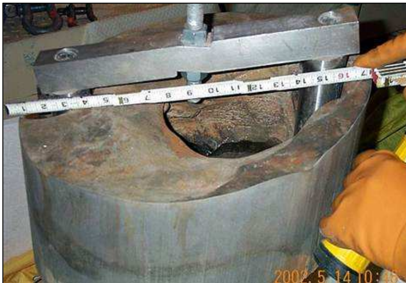
Fig. 6.5. The corroded part of vessel head after it was cut out from the rest of the vessel head.
