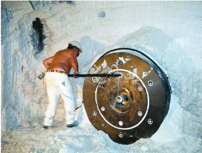
Figure 10.1. BAMBUS II experiment: Dismantling operation of the emplaced dummy canister in the Asse Research Mine (Bechthold et al., 2004)
